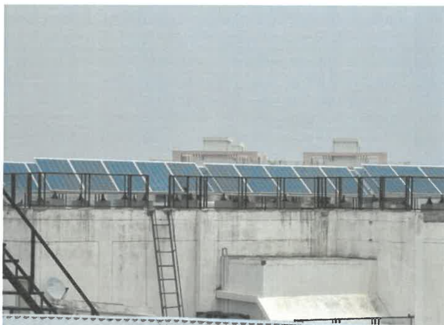
Picture 9: Solar panels
